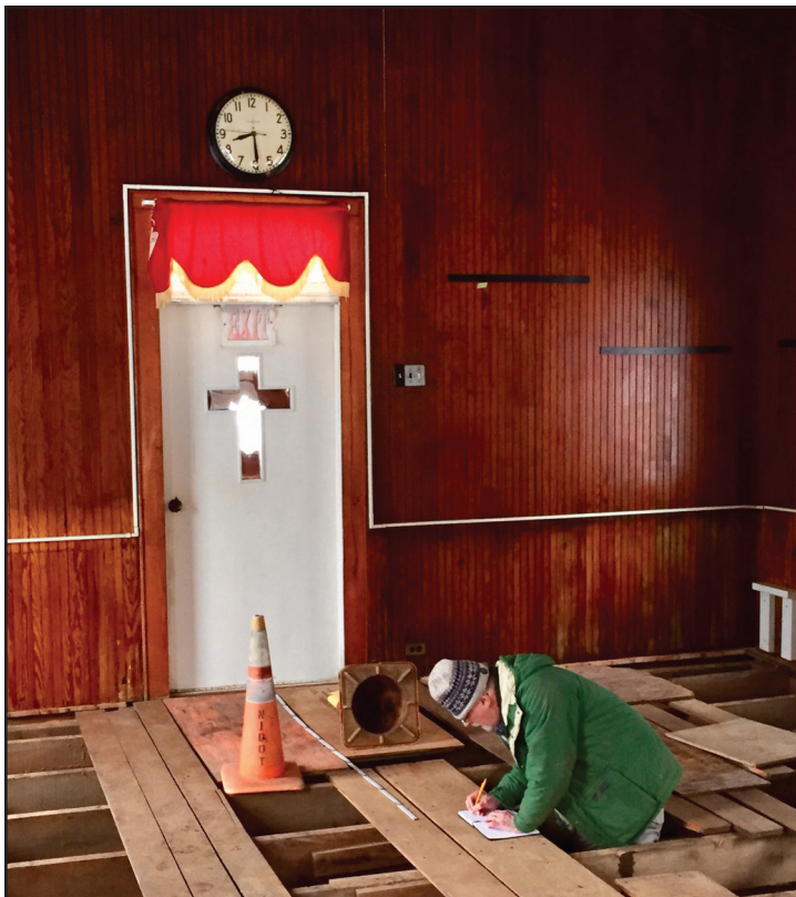
Board member and archaeologist, Ian Burrow, hard at work during the replacement of the main beam and restoration of the floor at Mt. Zion AME Church.
